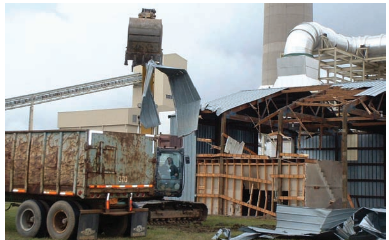
Demolition crews are changing their techniques to recycle more material and save money (photo courtesy WasteCap).
